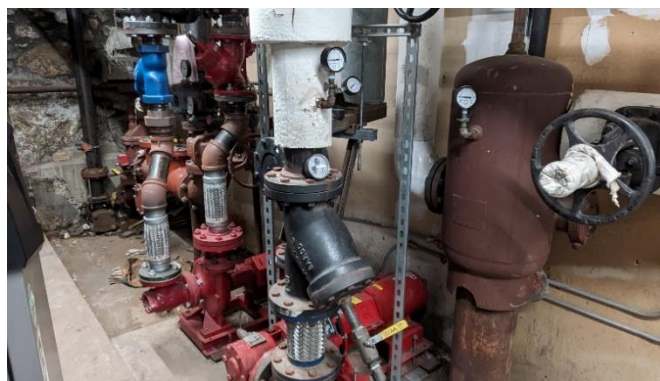
Existing Expansion Tank and Valves
