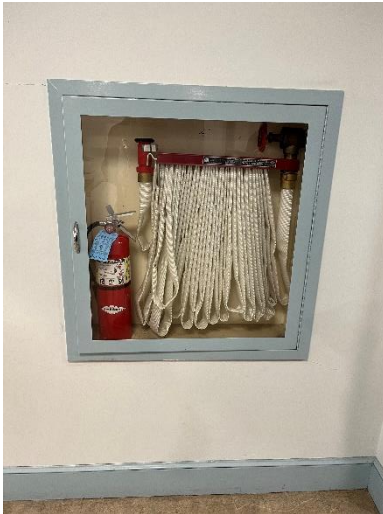
Fire hose connection
