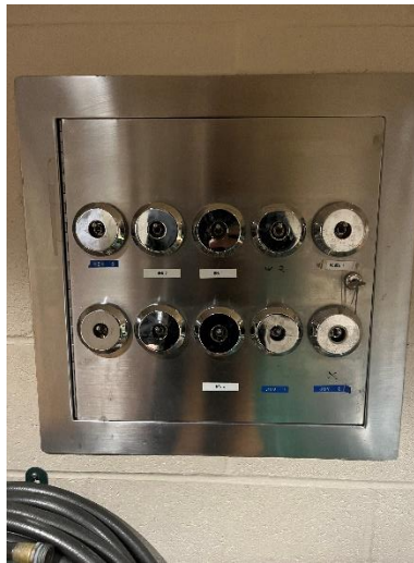
Cell fixture remote flushing
