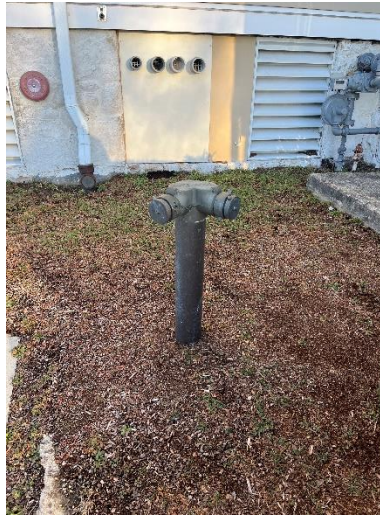
Fire Department Connection
