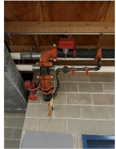
Sprinkler zone control valve assembly
