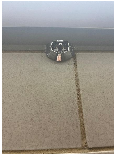
Institutional type sprinkler
