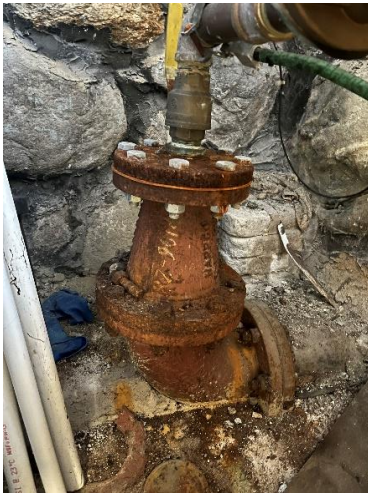
Domestic water service
