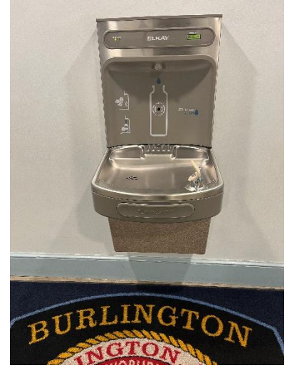
Electric water cooler
