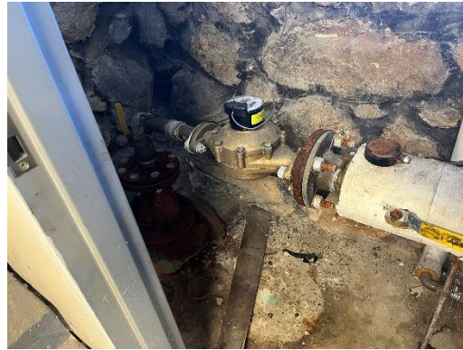
Domestic water meter
