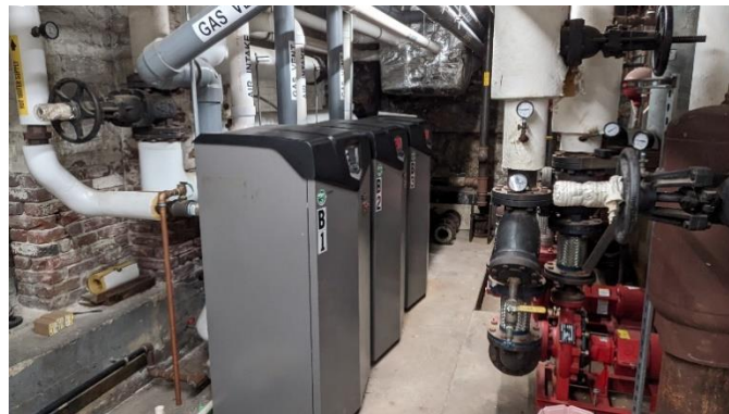
Existing Boiler Plant
