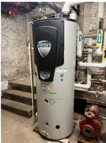
Domestic water heater
